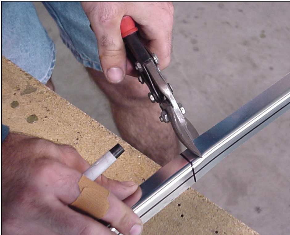
Cutting the “L” angle: Qty = 4 Layout: length = approximately 75mm. Rough cut: Snip both flange, twist to break off. Then do a final cut on the line.
